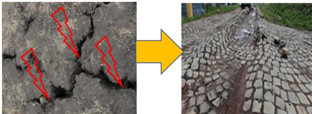
Figure 1 Behavior of the expansive soil and collapsed road section due to the unstable subgrade soil
